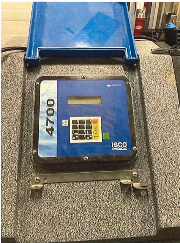
Isco 4700 composite sampler. Pump is good, refrigeration unit is bad.
