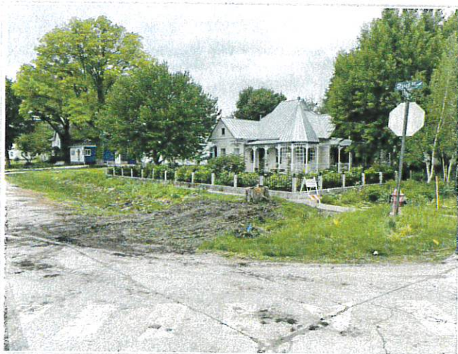
W Corner of 2nd & Rose Streets - MidAm dug out and backfilled at both corners to abandon gas pipe in the area
