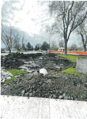
NE corner of site looking south, overview of the rain garden being backfilled and prepped for final F.E.S. and plantings
