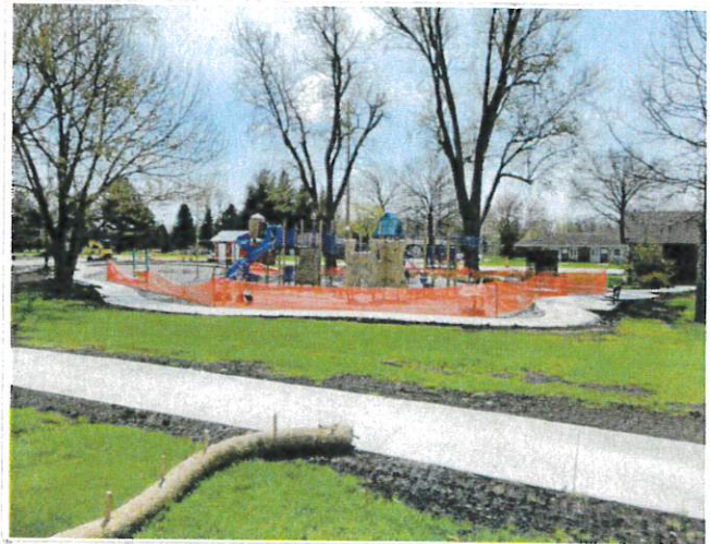
Looking south at the park, shows playground area being protected with construction fencing
