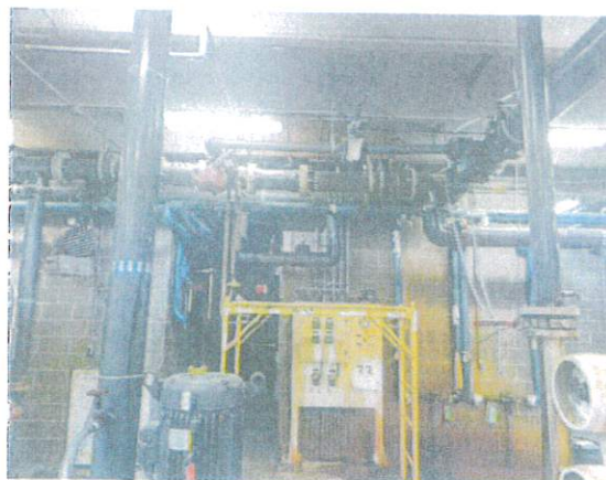
Feedwater/Total Permeate Monitoring & Sampling Panel
