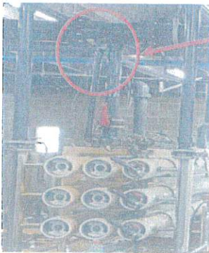
RO #1 Train- 4" sch80 PVC Permeate pipe into the 6" sch80 PVC Common Permeate Heading pipe is cracked at the Tee insert.
