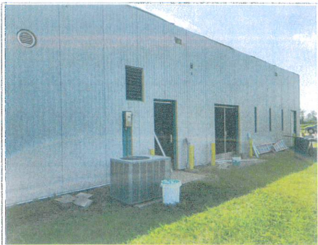
Overview of the north face shows crews working around miscellaneous items and trimming needed
