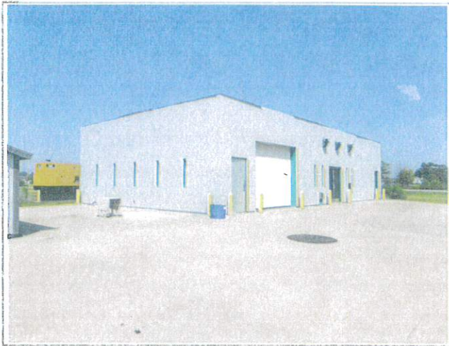
Overview from SW corner of site, shows panel install is complete with trims, caulking, coping and re-installation of lighting and signage left.
